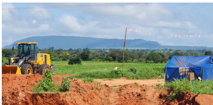
◀ Figure 4: The construction of a road towards the EACOP camp in Kimana village.
