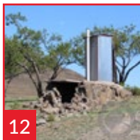
IMAGE 12 Dwellings alleged to have been damaged by mine blasts from the Letseng Mine, Maloraneng village, Mokhotlong, Lesotho 2018 Photo credit: Centre for Investigative Journalism, Lesotho
